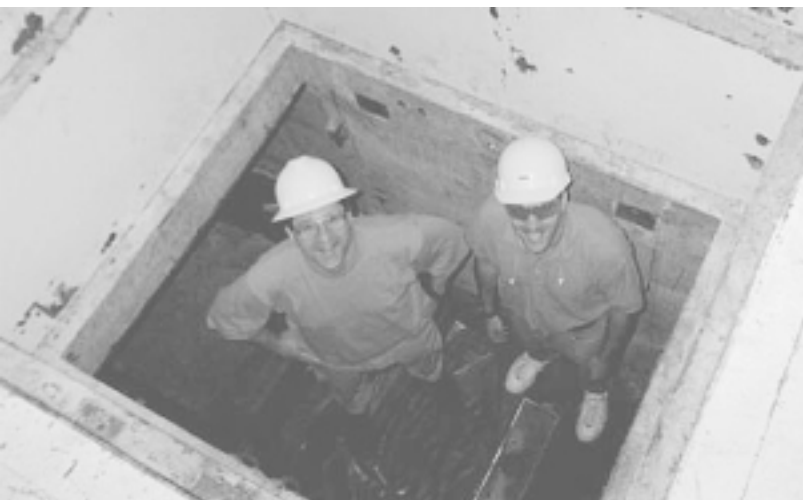
Mark Granus, left, project manager with Duke Engineering Services, and Scott Wendt, former reactor manager, stand in the cavity of the reactor core.
