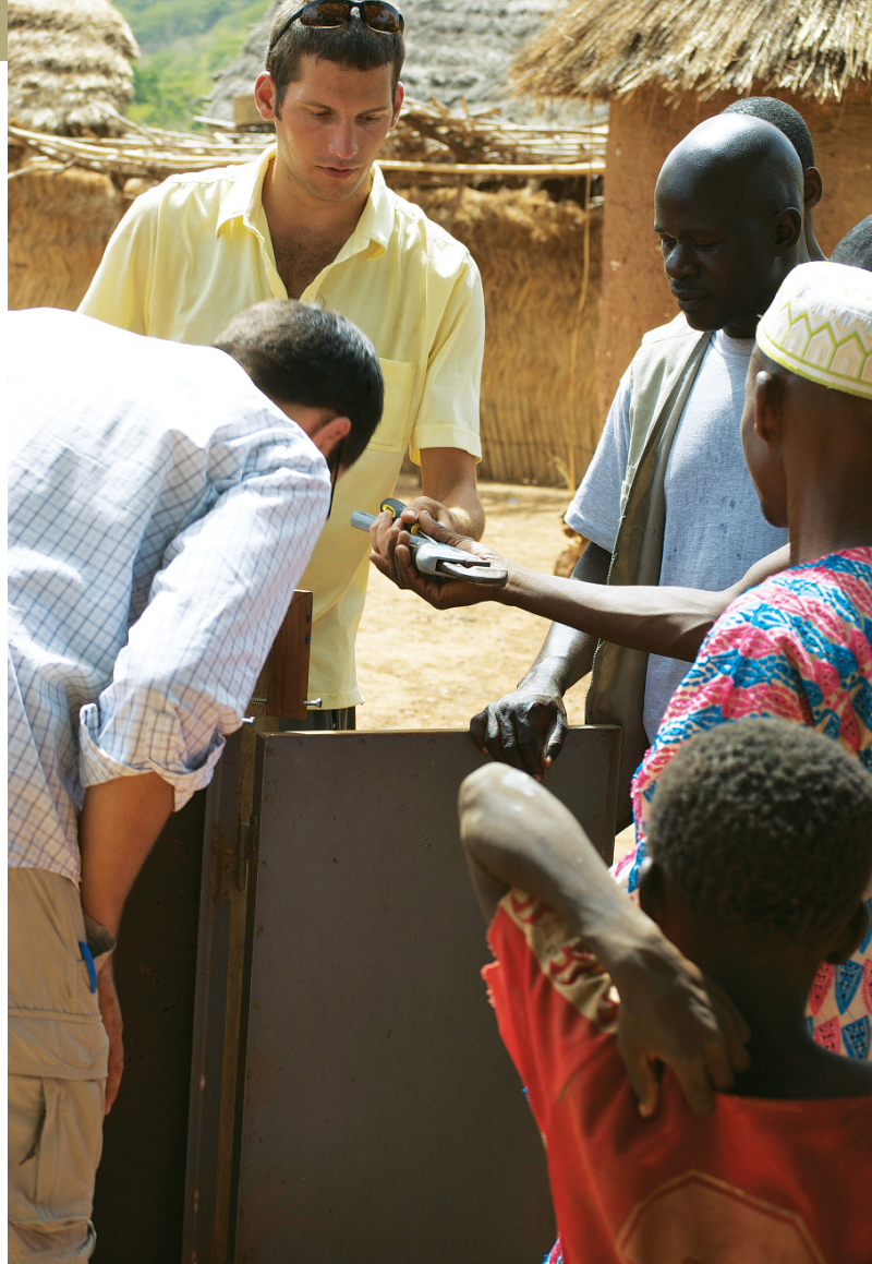
Wes Meier, a 2008 ME graduate, works with rural Malians to install a water valve.
